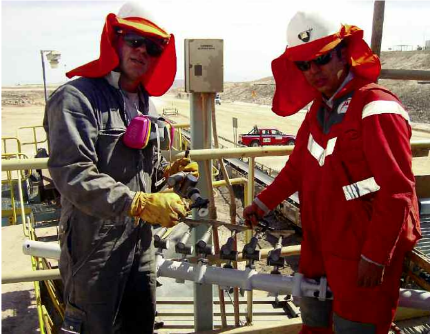
Heat and high altitude: the grueling conditions during the installation work in Chile ...
