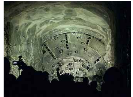
The breakthrough after almost five years: “Big Becky” finally sees light at the end of the tunnel; Photo: www.niagarafrontier.com
